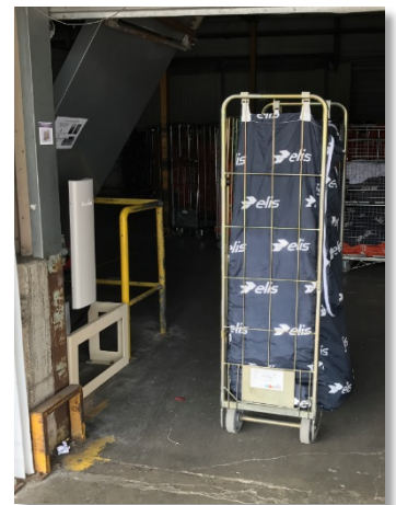
- Receiving area with xPortal RAIN RFID reader -
